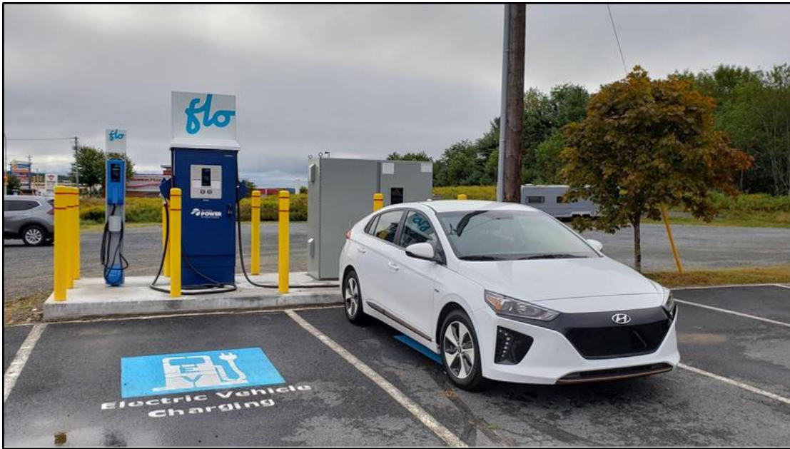
Figure 3: Typical EV Charging Location.
